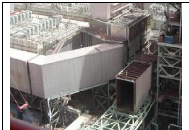
Figure 4. Large power plant duct supported on steel frames.
