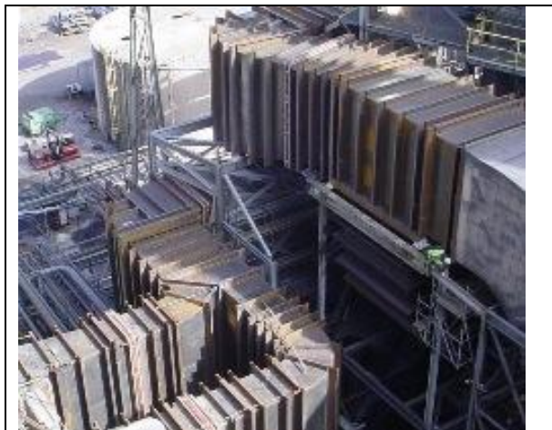
Figure 3. Large power plant ductwork routed through existing constraints.
