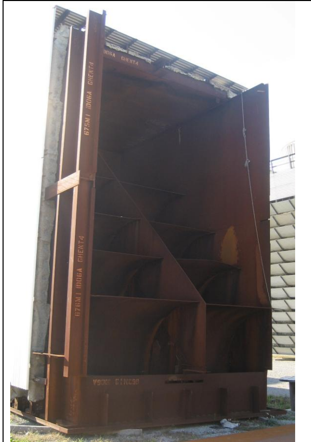
Figure 15. Turning vanes installed in a duct elbow.
