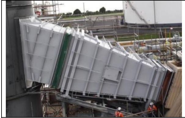
Figure 20. Flow energy can be regained by using verified evase designs following fans.
