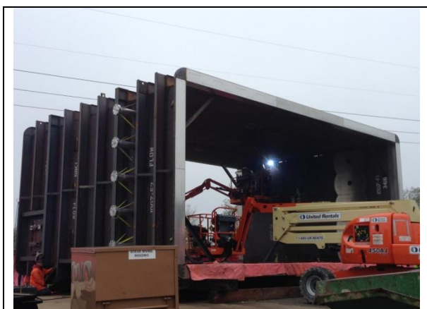
Figure 25. Large duct section being assembled prior to installation. Notice the alloy cladding on the expansion joint frame and at the test portson the far side of the duct. Also notice this duct section was shipped in flat panels since the welding is occuring in the corner of the duct.
